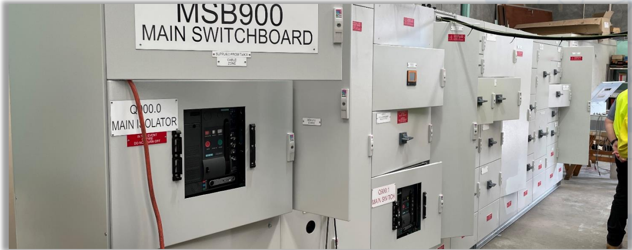
Main PPF electrical switchboard complete
