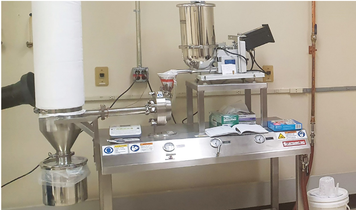
Alpha's dedicated jet mill installation – Binghamton, USA
